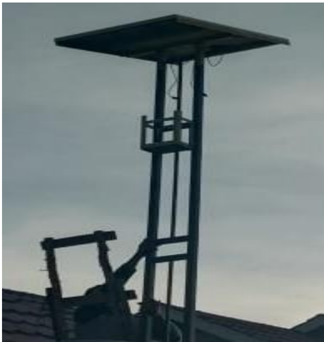
Figure 2. Installed Solar Panel
