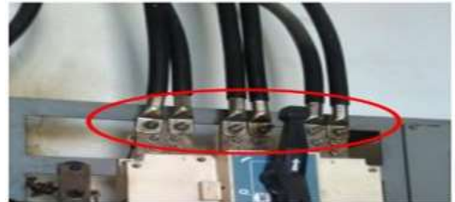
Figure 1. Incoming Unit LVSDP [2]
