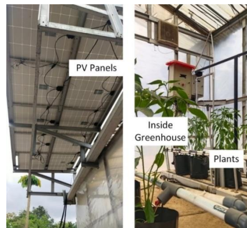
Figure 2. The PV systems installed on solar-powered greenhouse considered in this study.
