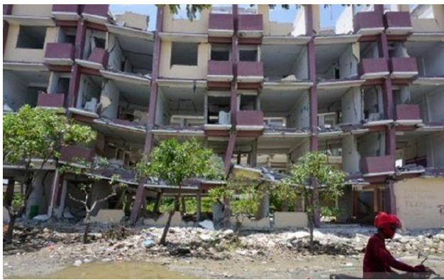
Figure 1. Flat buildings damaged by the earthquake in Palu, Central Sulawesi
