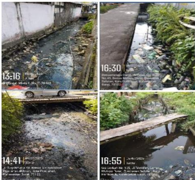
Figure 2. Condition of Several Existing Channels at the Research Location
