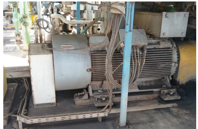
Figure 2.3 Motor Coal Mill 2B 6P-2343-RM-B
