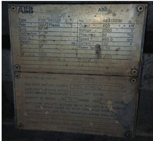
Figure 2.3 Motor Coal Mill 2B 6P-2343-RM-B Specification Data
